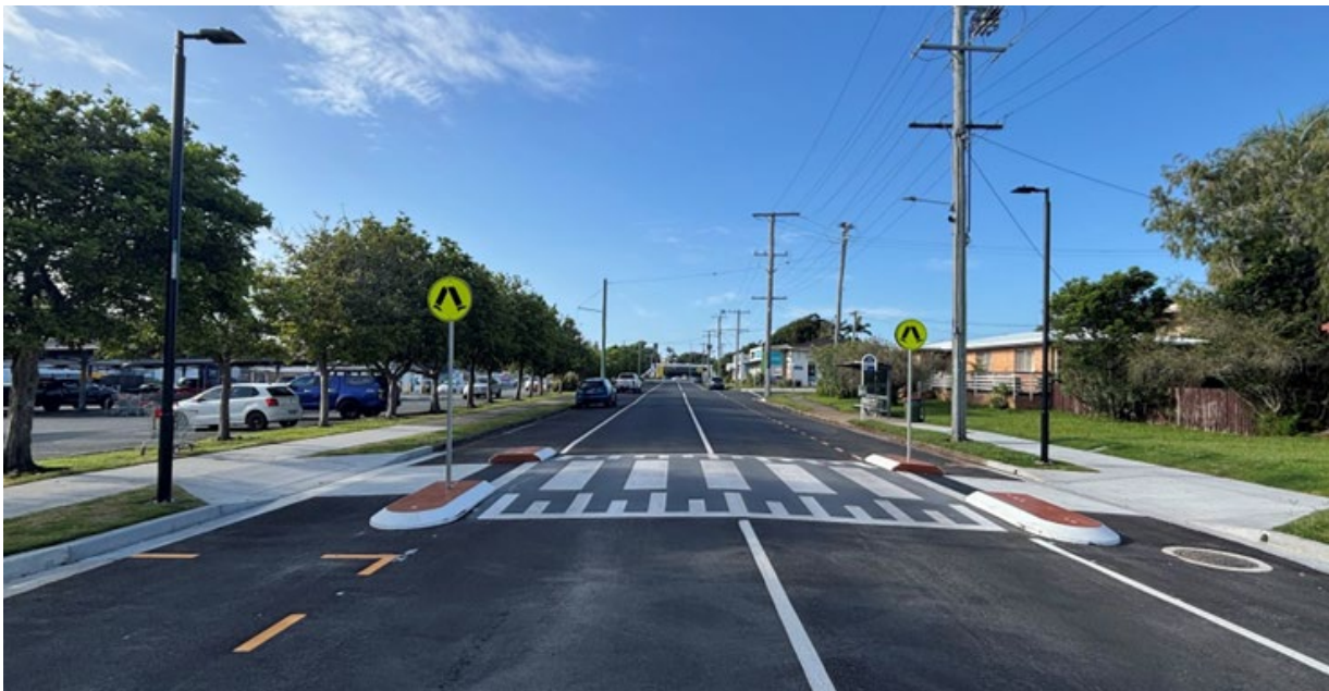
Figure 4.4 – Raised crossing incorporating separation devices and kerb and channel to facilitate drainage
