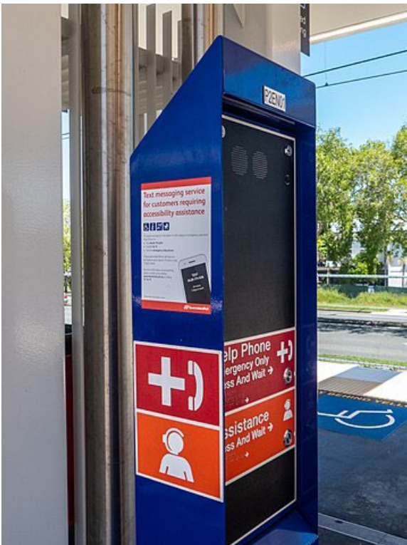
Figure 153 Platform help phone, Yeronga rail station
