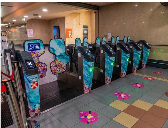
Figure 85 Fare validators and accessible fare gate, Roma Street rail station
