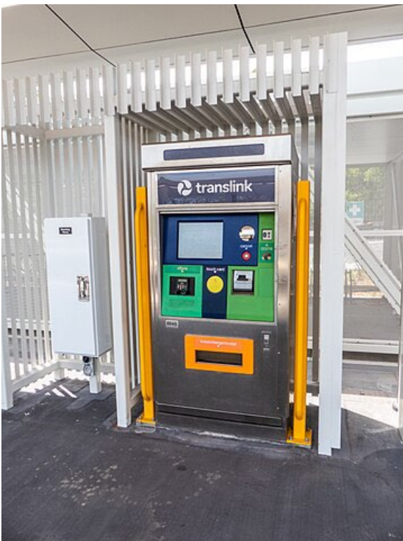
Figure 88 Add Value Vending Machine, Fairfield rail station
