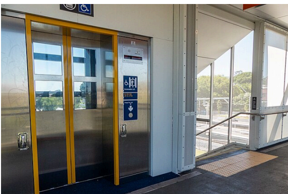
Figure 177 Vertical transport, Yeronga rail station
