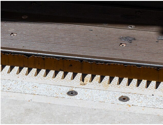
Figure 74 Platform gap filler and treadplate, Yeronga rail station
