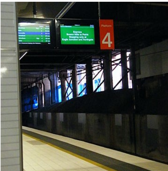
Figure 160 PIDs, Fortitude valley rail station
