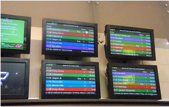
Figure 152 PIDs, Fortitude Valley rail station
