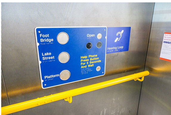
Figure 185 Lift controls, Yeronga rail station
